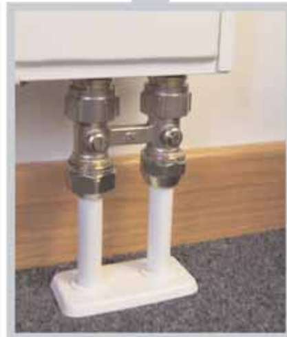
Isolation valves on supply and return piping
